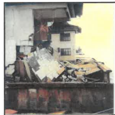
Hurricane Elena Damage 1985
