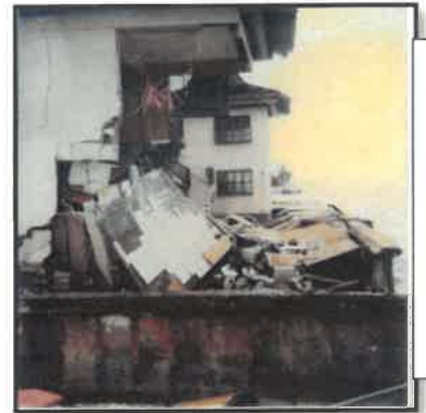
Hurricane Elena Damage 1985
