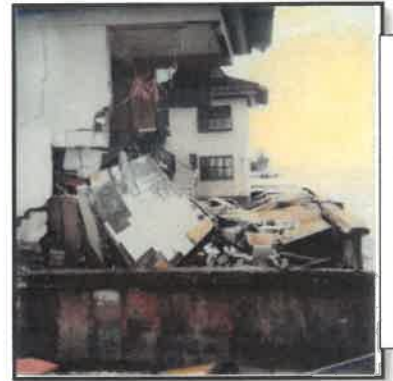
Hurricane Elena Damage 1985
