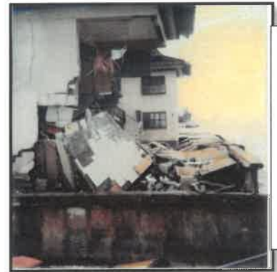
Hurricane Elena Damage 1985
